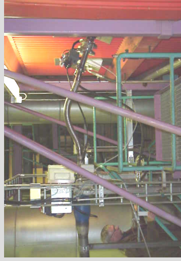
Bioma| burner connected to the boiler.
